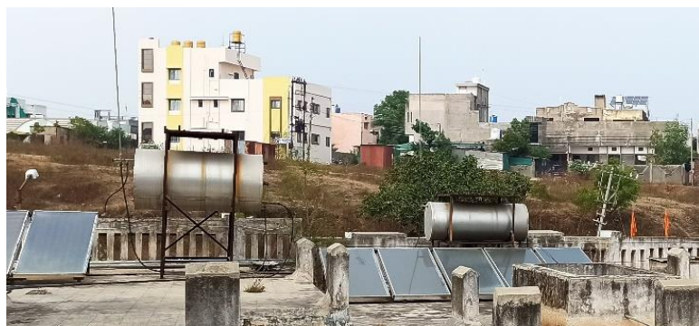
Figure 15: Solar panel and water heater on the roof of SDH Karanja
