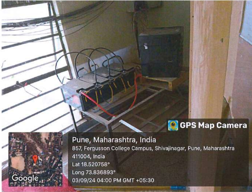
UPS in UGC Building
