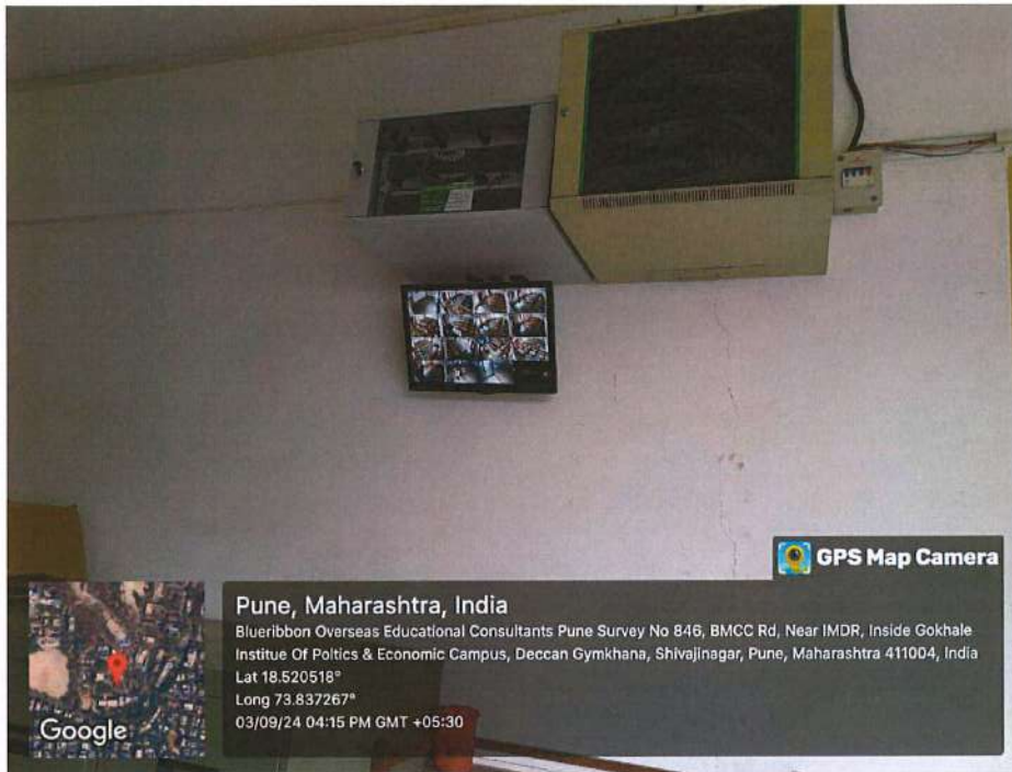
CCTV & Switch Academic Building
